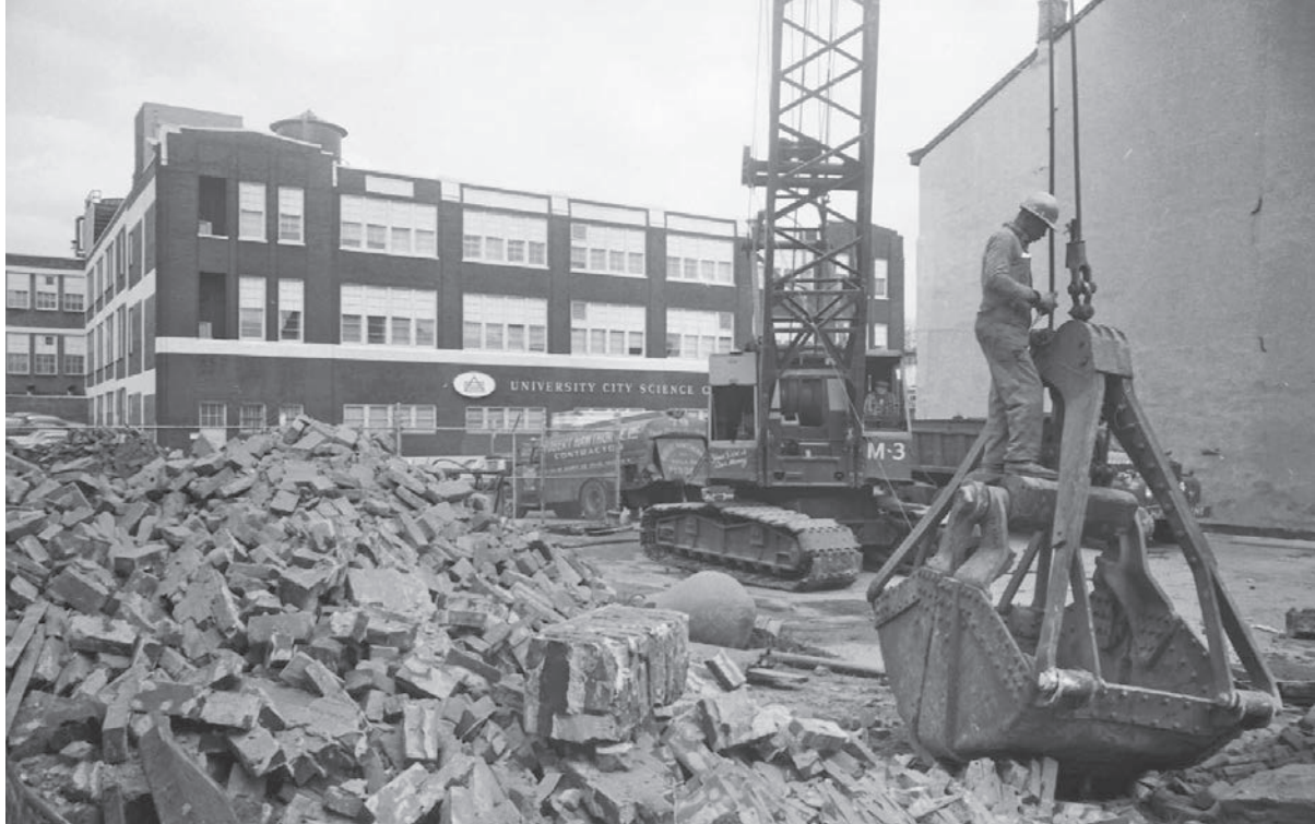
Demolition of a building near the southwest corner of 34th and Market streets, 1967. In background, the Science Center headquarters building on the north side of Market. In January 1965 the Science Center Corporation acquired the building from the Stephen Greene Company, a printing firm. Collections of the University Archives and Records Center.
